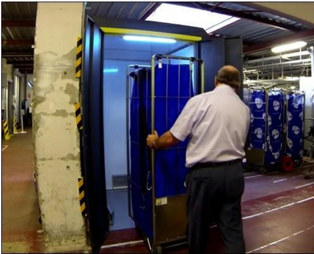
To track clean linens, BIH installed an RFID reader and antennas in a reading cabin resembling a freestanding wardrobe.
